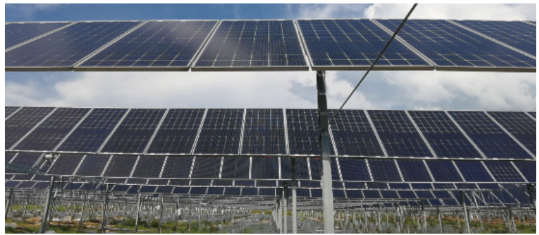
Figure 32 Mengxu 200 MW PV power plant in Yuchai, Guangxi, China
