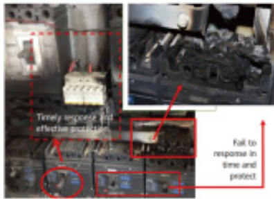
Figure 18 Case 1: DC circuit breaker failure
