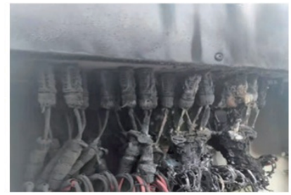
Figure 20 Case 3: Burnt DC terminals due to overtemperature
