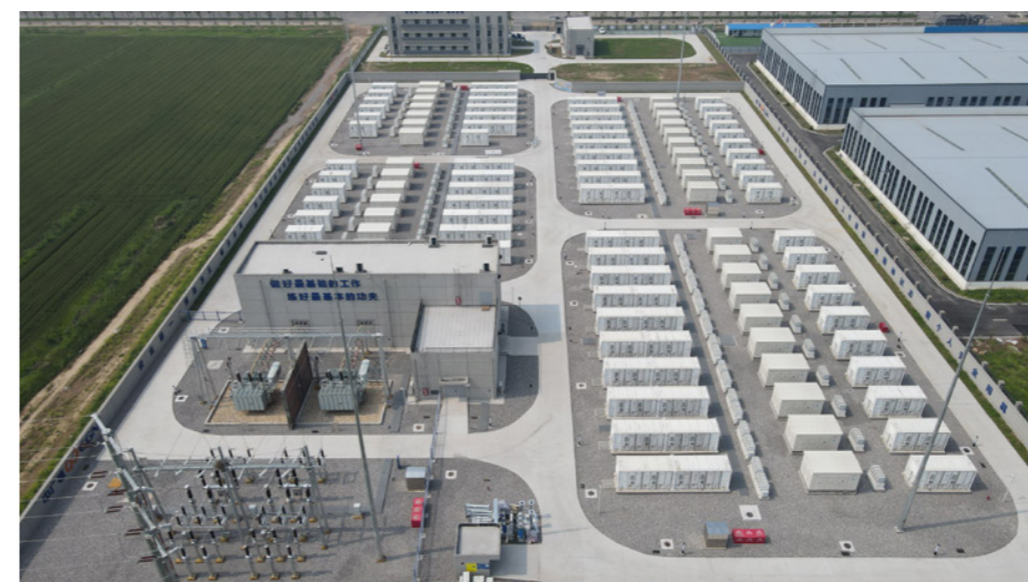
BESS project in Hubei Province, China
