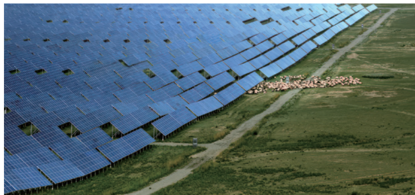
Hainan 2.2GW High DC PV Plant @Qinghai Province
