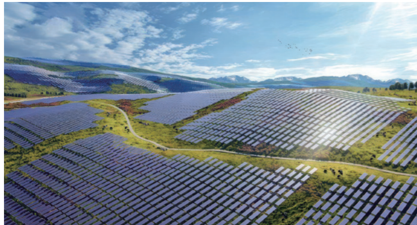
Yalong River 1GW Keda PV Plant @Sichuan Province
