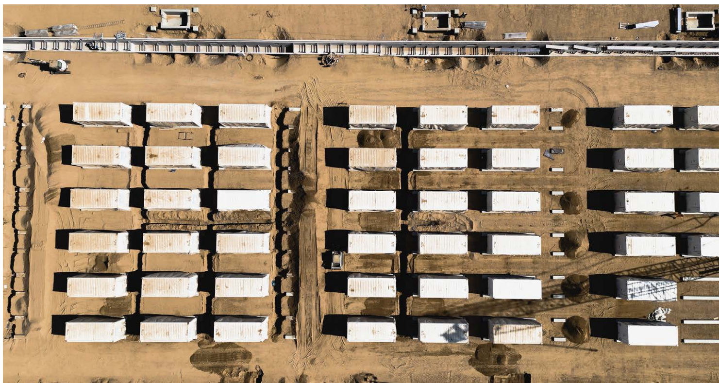
FusionSolar Smart String ESS installed at the Red Sea project. In this harsh desert environment, the BESS will have to deal with high temperatures, as well as humidity and salinity.
