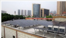
PetroChina Gas Station with optimizers (120 kW)
