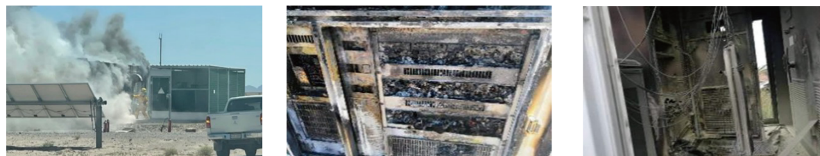
Figure 18 Inverters and combiner boxes on fire due to DC short circuits
