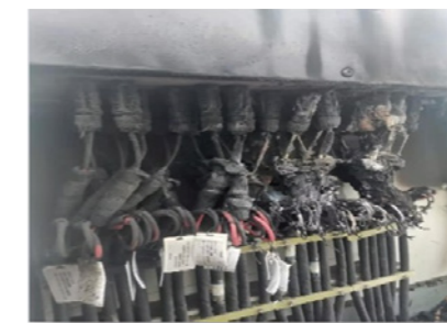
Figure 17 Fire caused by terminal overtemperature
