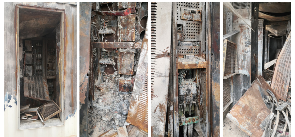
Figure 11 Fire caused by inverter insulation failure
