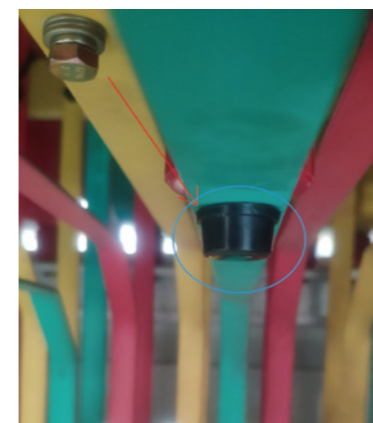
Figure 28 Insulation protection solution for branch buses of low-voltage cabinets
