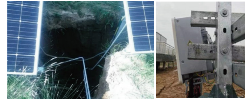
Figure 15 Poor contact of terminals due to land subsidence
