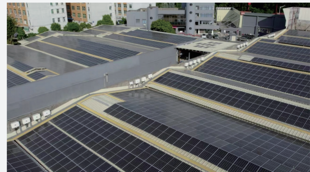
▲ Figure 5-2: Max Li-Power building a distributed PV plant for Qingchuang Meiju in Shenzhen
