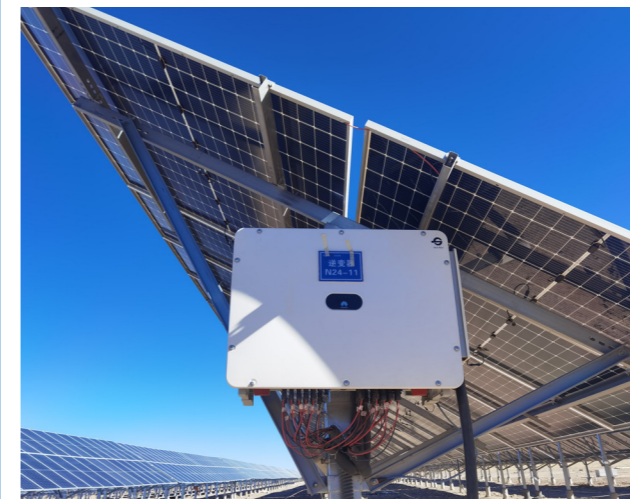
▲ Figure 6-2: Huawei inverters work well in high altitude project
