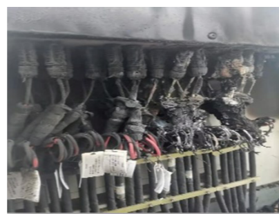
> Fire caused by connector overtemperature
