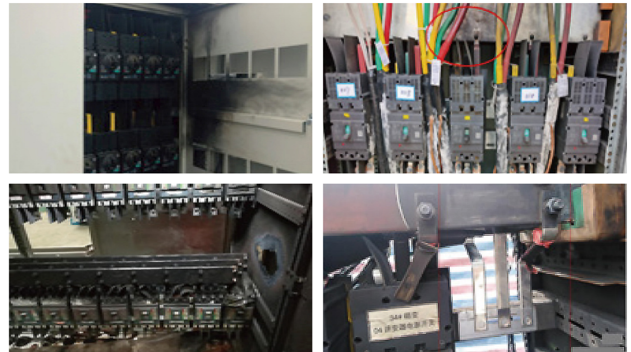
> Safety incident caused by arcing at a transformer station
