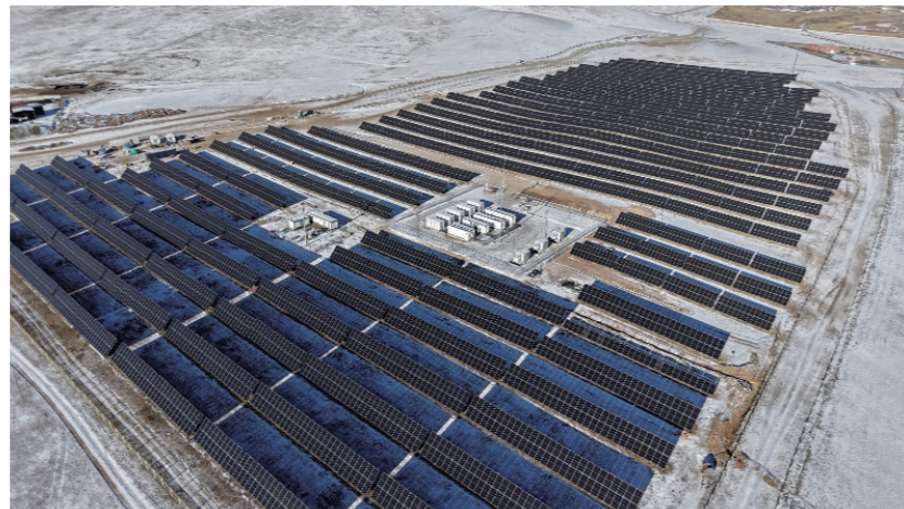
Figure 3-2: Mongolia MAK 53.7 MW PV + 139.5 MWh ESS coal mining microgrid project
