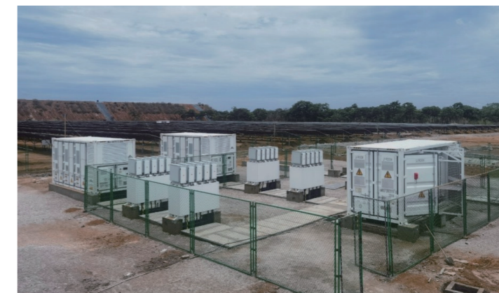
Figure 3-1: M mine 18 MW PV + 10 MWh ESS copper mining microgrid project
