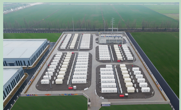
A 100MW BESS in China's Hubei project used Huawei's battery risk warning function
