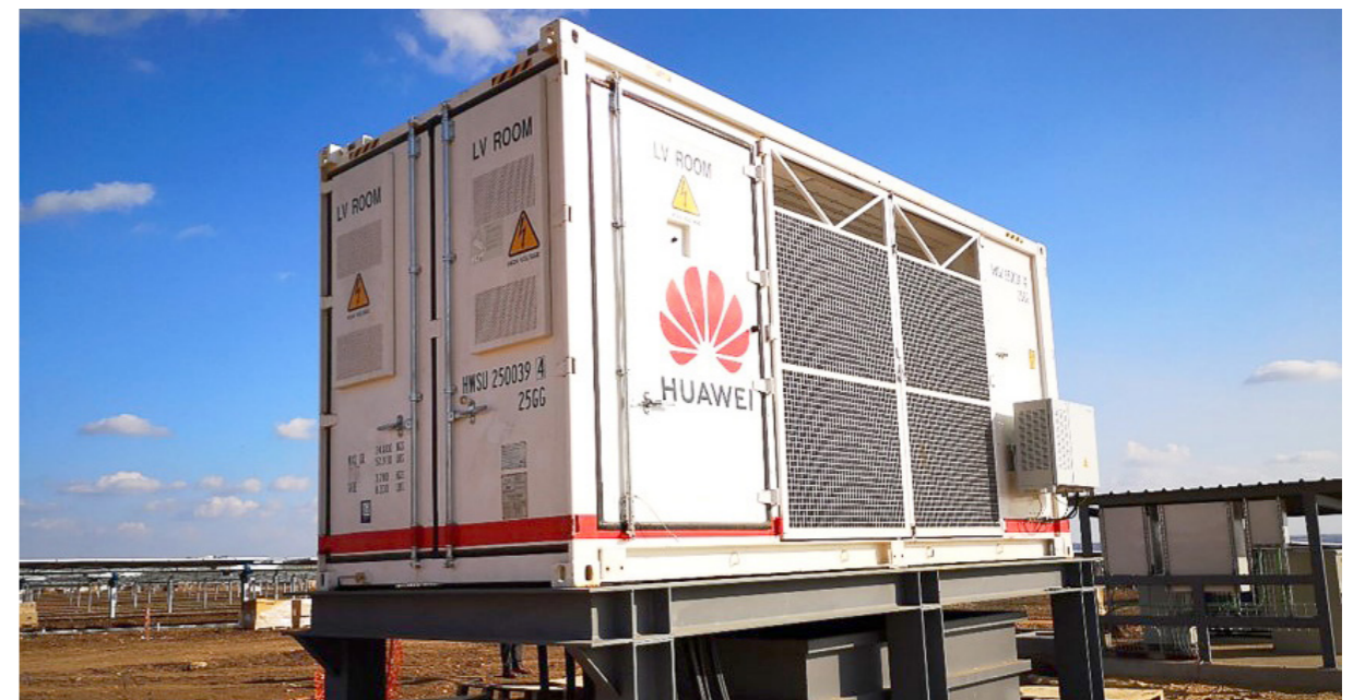
> A 26 MW PV project in Spain
