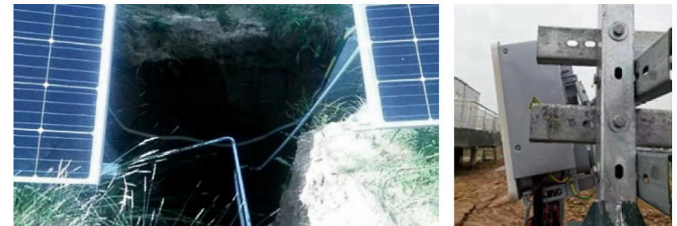
> Poor contact of connectors due to land subsidence
