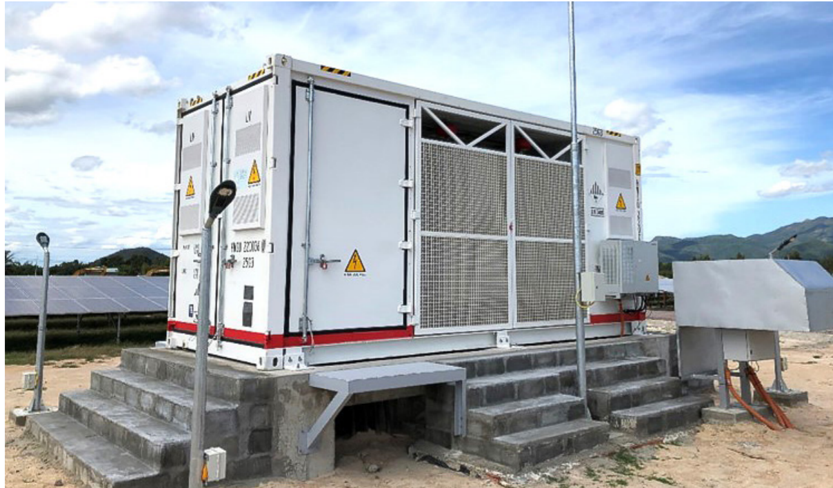
> A 50 MW PV project in Vietnam
