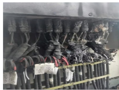
> Fire caused by connector overtemperature
