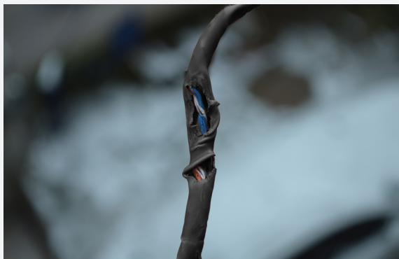
DC power cable is damaged
