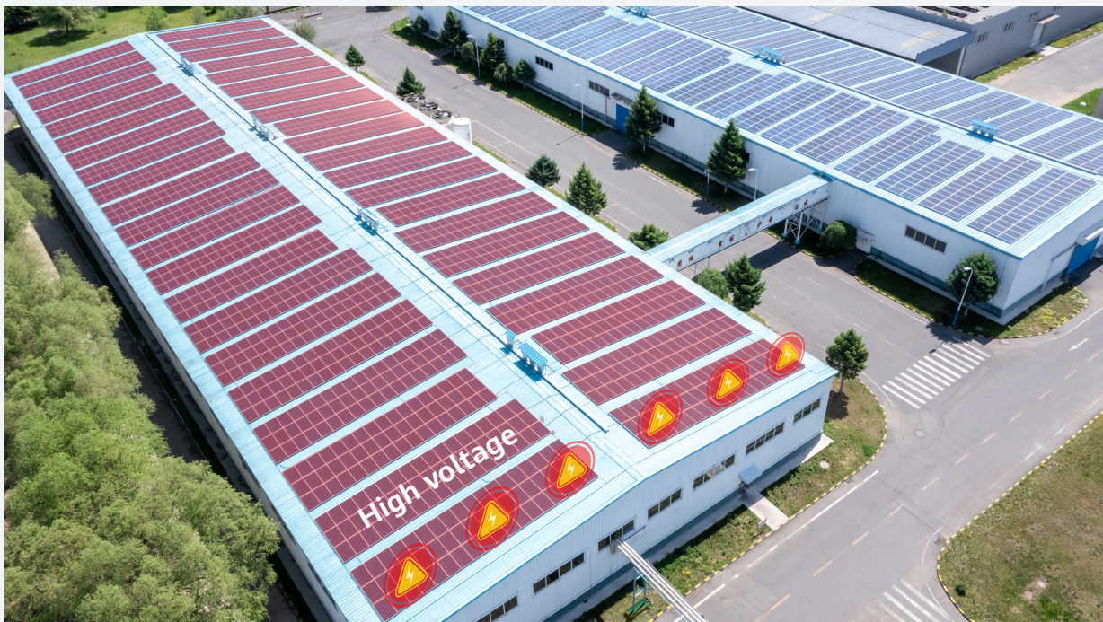
Figure 9. High voltage on the rooftop
