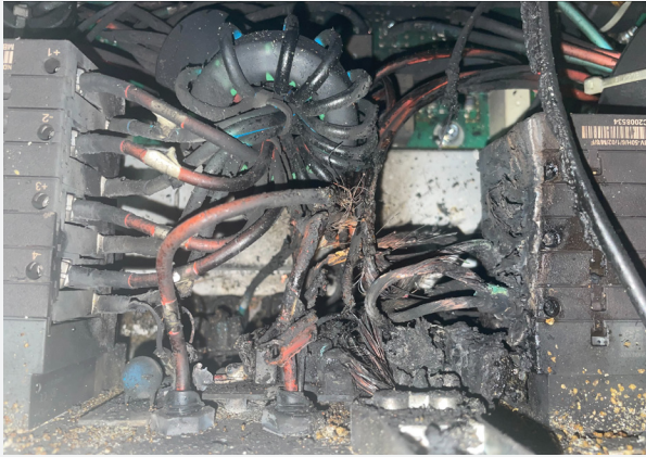
Burned DC cables
