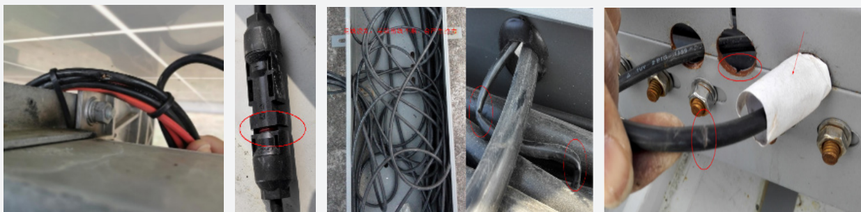
Cables tied to a support
