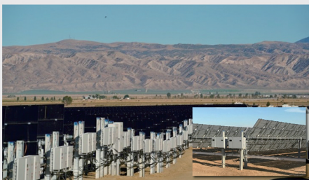
43 MW Ground-Mounted Smart PV Plant, Cuyama, California, USA
